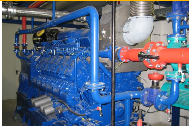
Combined heat and power plant Oelper
